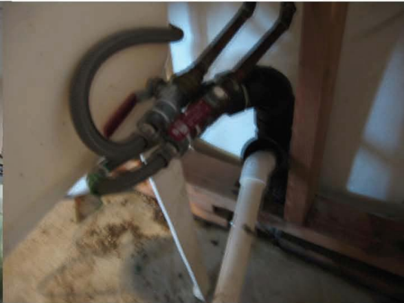
Drain out to sewer
